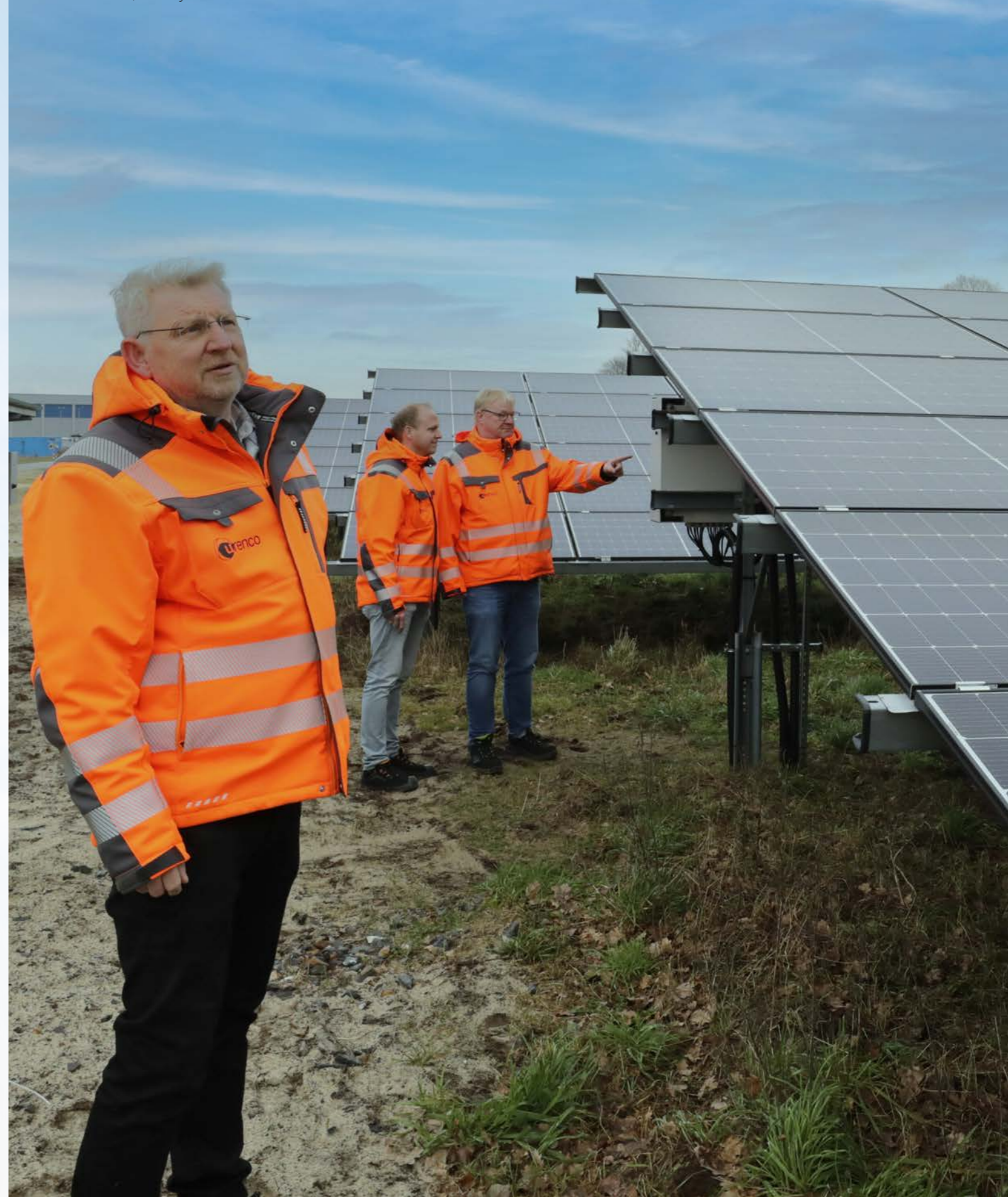
New solar park installation Gronau, Germany.
